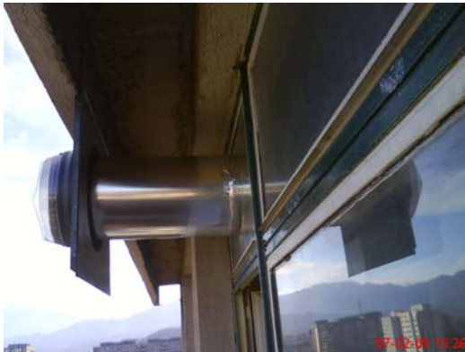
Fig. 2 Daylight dome collector of the horizontal SUNPIPE installed on the façade
