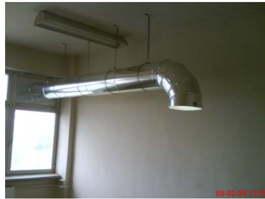
Fig. 3 Horizontal SUNPIPE ending with two 45 degrees elbows above imaginary false ceiling
