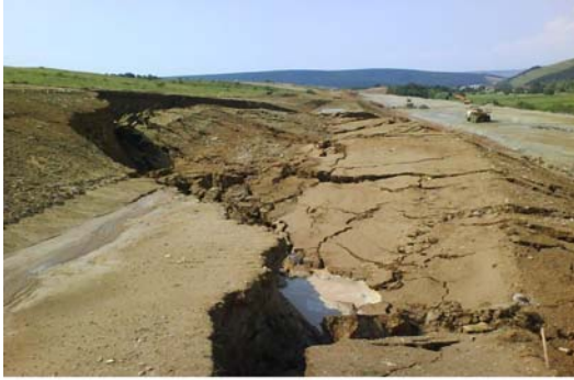
Fig.5 Sliding km 45+700 – km 45+780
