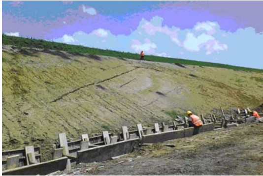
Fig.2 Cracks that occurred during the excavation for the longitudinal drain
