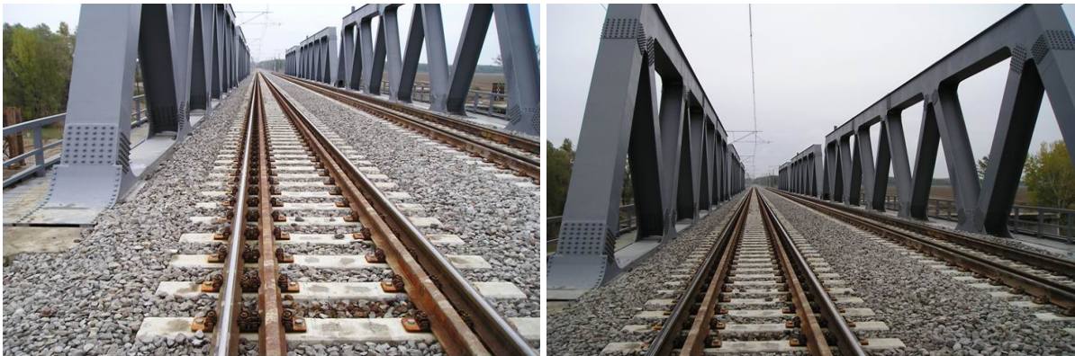
Figure 13. Pan European Corridor IV, Bucharest North - Campina Section, railway bridge over the river Prahova, Rail and guard rail Vossloh KS with Skl 12 fastening system
