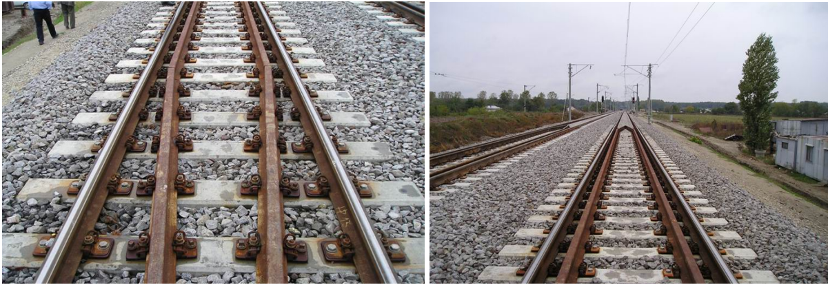
Figure 14. Pan European Corridor IV, Bucharest North - Campina Section, railway bridge over the river Prahova, Rail and guard rail Vossloh KS with Skl 12 fastening system
