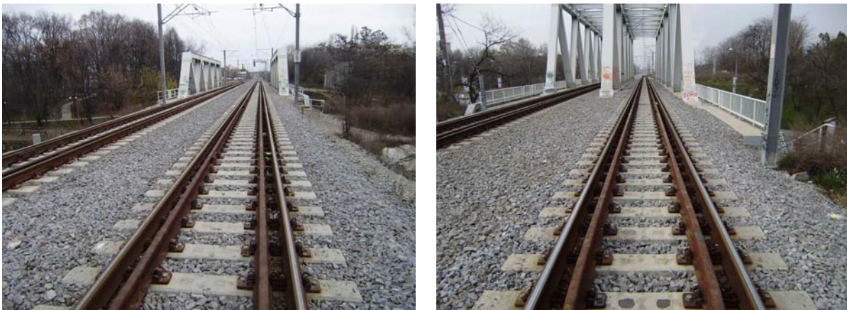
Figure 17. Pan European Corridor IV, Bucharest - Constanta Section, Miorita Baneasa Bridge over National Road 1, Rail and guard rail Vossloh KS with Skl 12 fastening system
