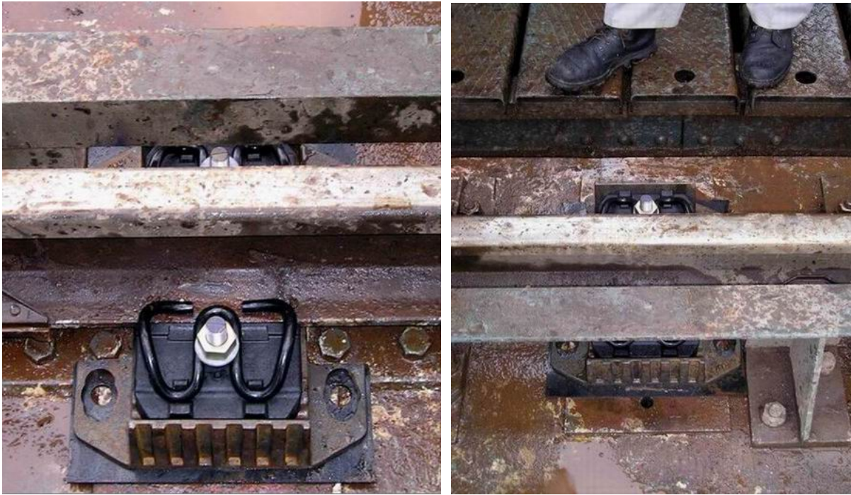
Fig. 12 The Vossloh DFF 300-1 system installed on Danube – Cernavodă bridges
