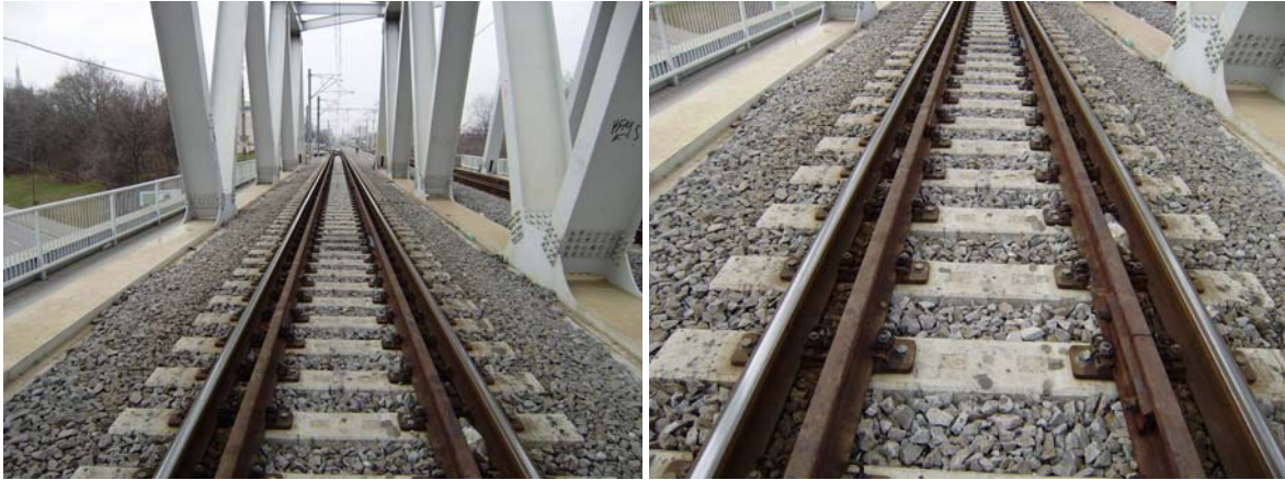
Figure 16. Pan European Corridor IV, Bucharest - Constanta Section, Miorita Baneasa Bridge over National Road 1, Rail and guard rail Vossloh KS with Skl 12 fastening system
