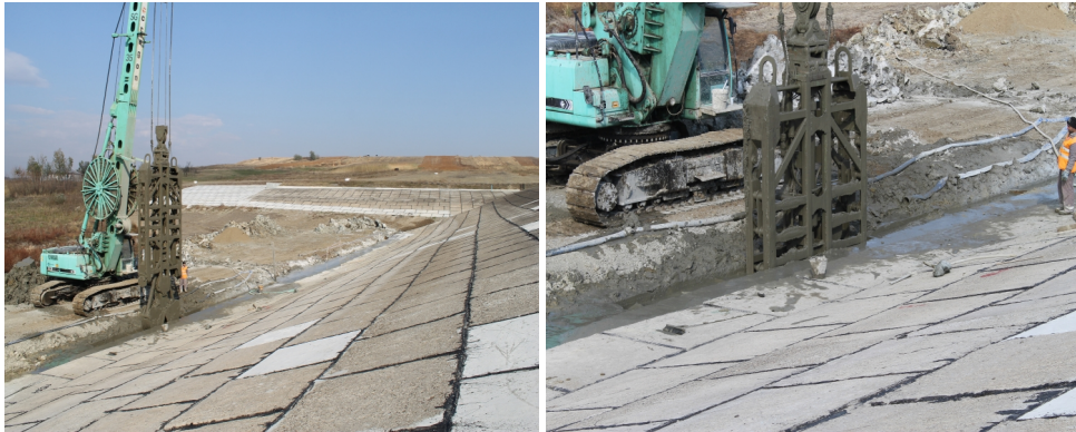
Fig. 1. Aspects from the execution of the sealing screen at Mileanca dam – Excavation of a panel using specialized installation type Kelly
