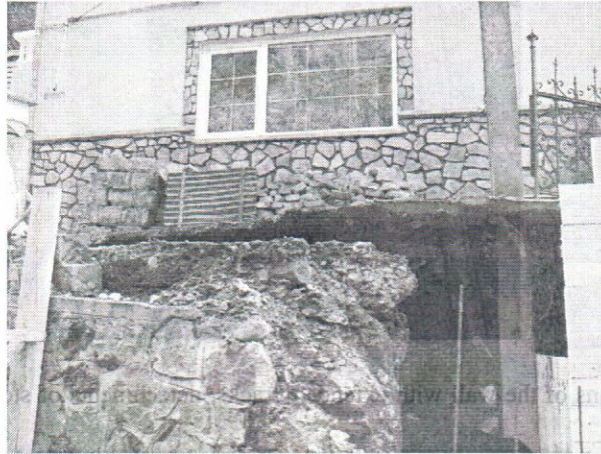
Fig. 5. – Portion of the wall detached from the wall.
