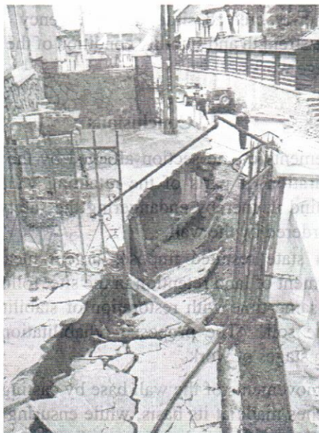
Fig. 6. – Crashing of portions of land behind the retaining wall.
