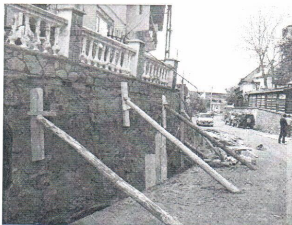
Fig. 2. – The digging carried out on long sections near and under the foundation quota of the retaining wall.
