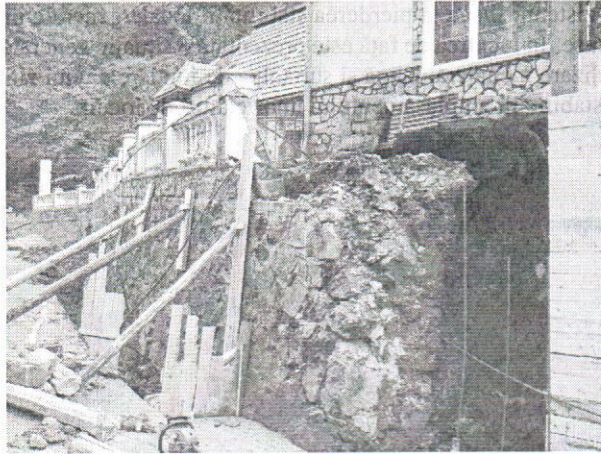
Fig. 8. – Blocking the movement of the retaining wall (using concrete works) and sustaining its wall parament.
