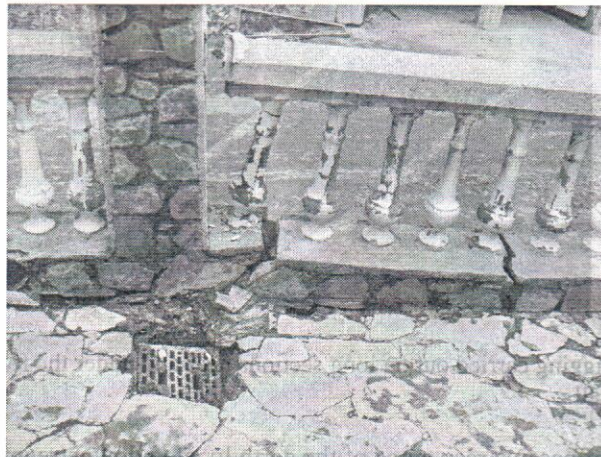
Fig. 4. – Cracks in the protection bulwark area.
