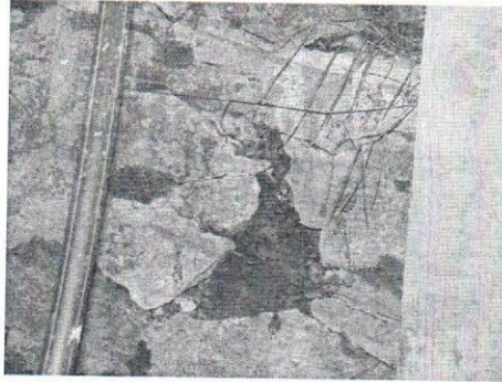
Fig. 7. – Portions of the wall with extended cracks, detachments of stone and abundant vegetation.
