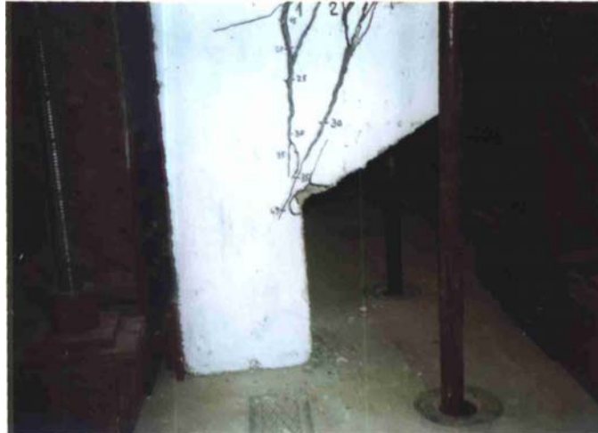
Fig. 5 Crushed concrete at the lower corner of console-column junction
